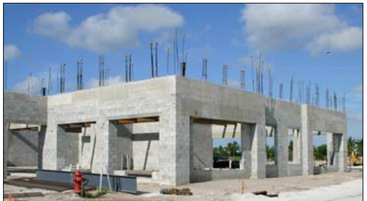
Crews work at the Canyon Town Center site in suburban Boynton Beach. There will be an Italian restaurant in the retail/residential center.
